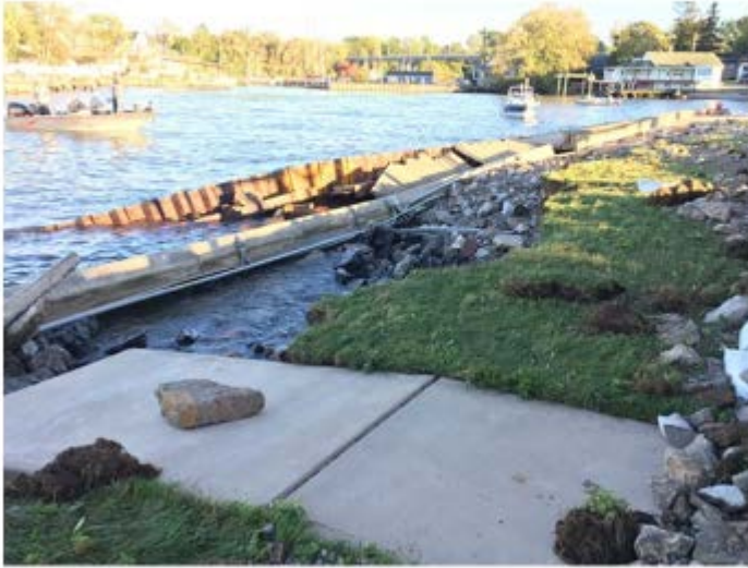
Retaining wall collapse at Olcott Yacht Club September, 2017 Photo: http://www.wgrz.com
