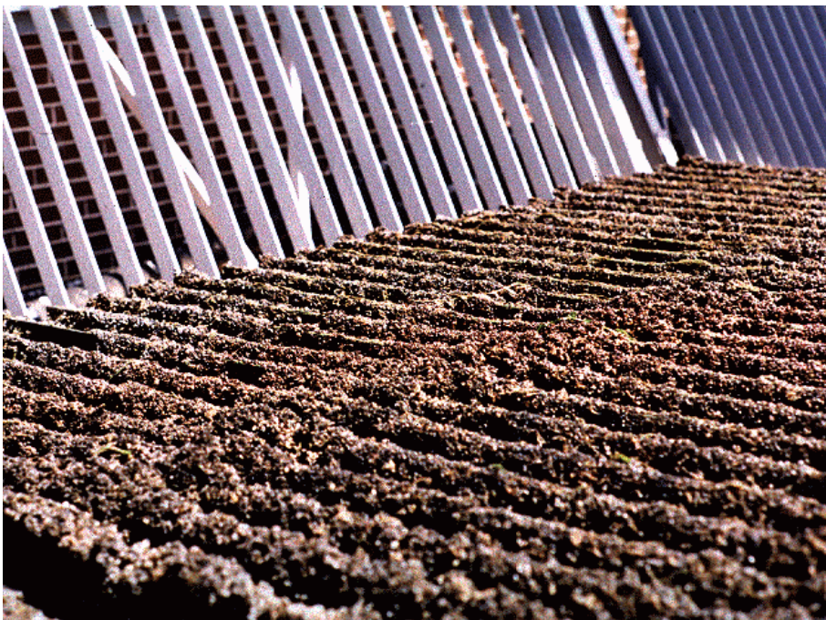
Figure 2 – Zebra mussel fouled trash rack
