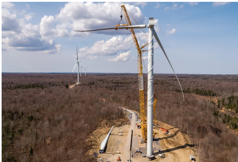
The Roaring Brook Wind Farm is a 79 MW capacity in Lewis County, New York constructed by The Wesson Group .
