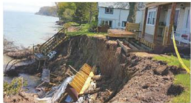
Coastal Infrastructure impacted by erosion in Monroe County. Image credit: Mary Austerman, New York Sea Grant. 2017 Coastal Flooding Survey Project
