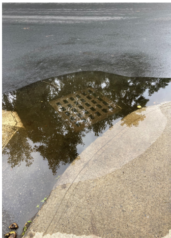
Storm drain back-up due to an extreme high tide. Credit: Jessica Kuonen
