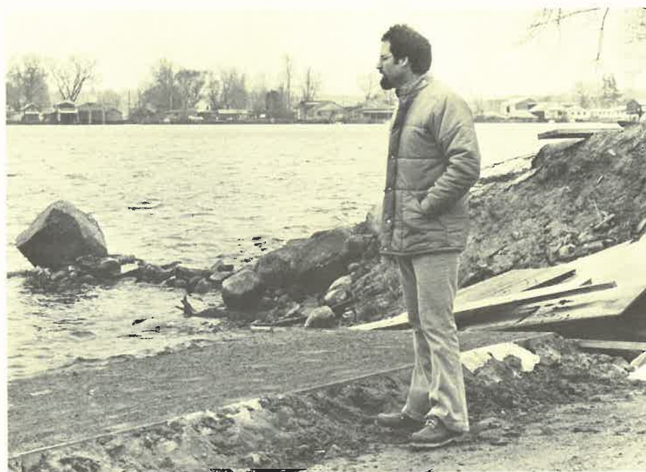
Mike Voiland (above) from Sea Grant's Brockport office looks over the construction of Sodus Point's new boat launch (pictured here) which helped to save the county of $44,000.
