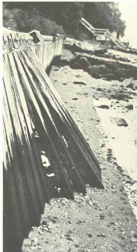
An example of undercutting, scouring and loss of backfill due to inadequate toe protection.
