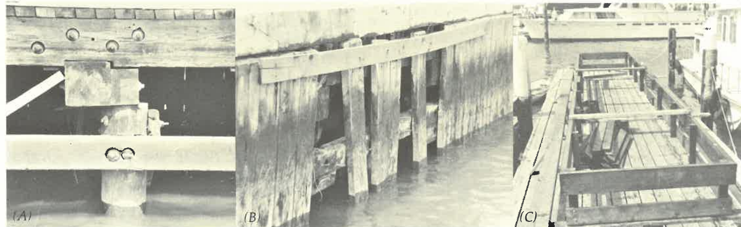
Repairing aging docks suffering from (A) slippage and (B) missing parts, and replacing old sections with (C) new construction are increasing management problems at New York City's public marina on 79th street — especially since federal funding may not be available in the future.
