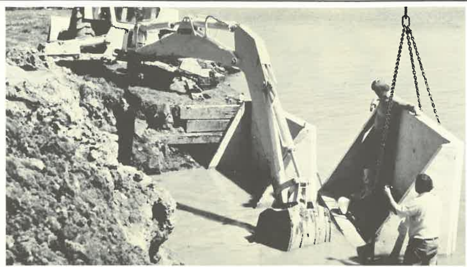
The design and construction of coastal structures often requires specialized marine technology.
