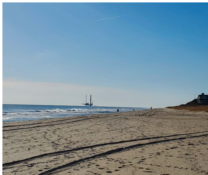
The construction vessel "Jill" marks the beginning of the construction and operations phase for South Fork Wind Farm offshore of Long Island. Photo: Gwen Gallagher/NYSG
